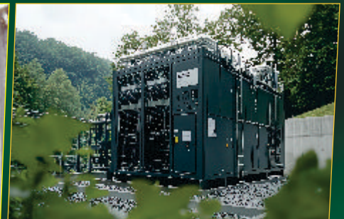
Power Backup for Common Areas
